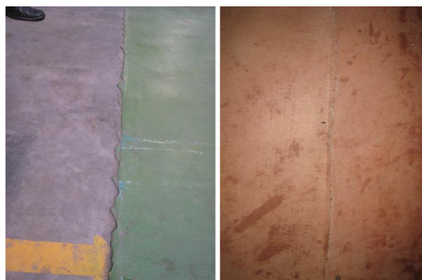
Bad coating end finishes
